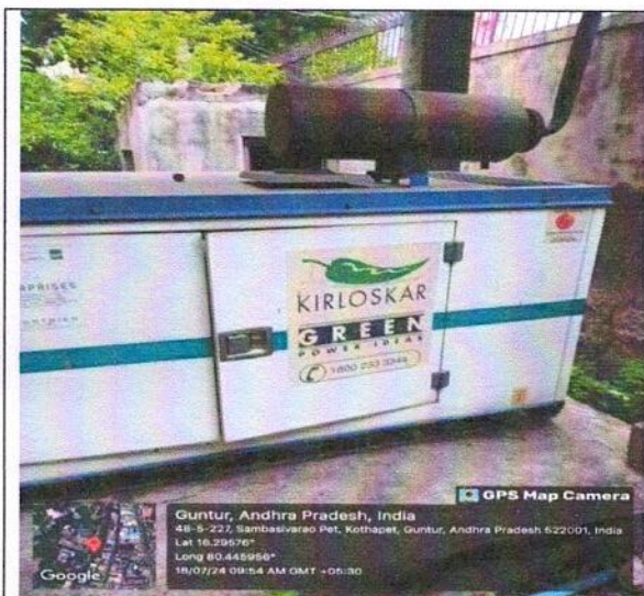
30 KV KIRLOSKAR Generator
